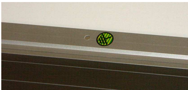
Grounding sign in detail
